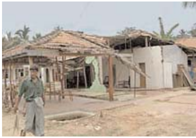
Destruction near beach in Tangalle
